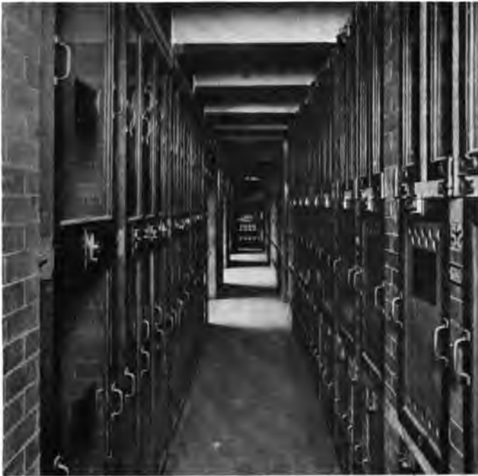
Fig. 1. High-Tension Equipment. (New York Edison Company.)
